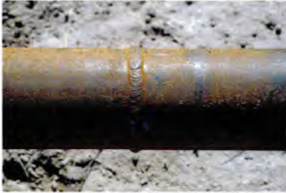
Close-up of pipe weld: Notice flash rusting.
