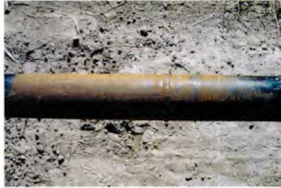
Pipe surface requiring field coating.
