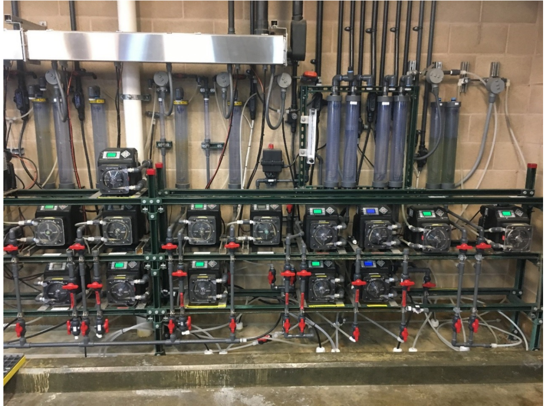
Figure 5 Chemical Feed Pumps
