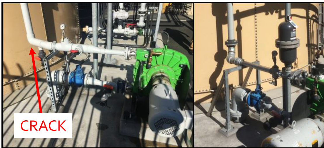
Figure 21 Sludge Pump Modifications
