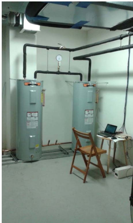
Figure 23. Water Storage Tanks and Data Logger
