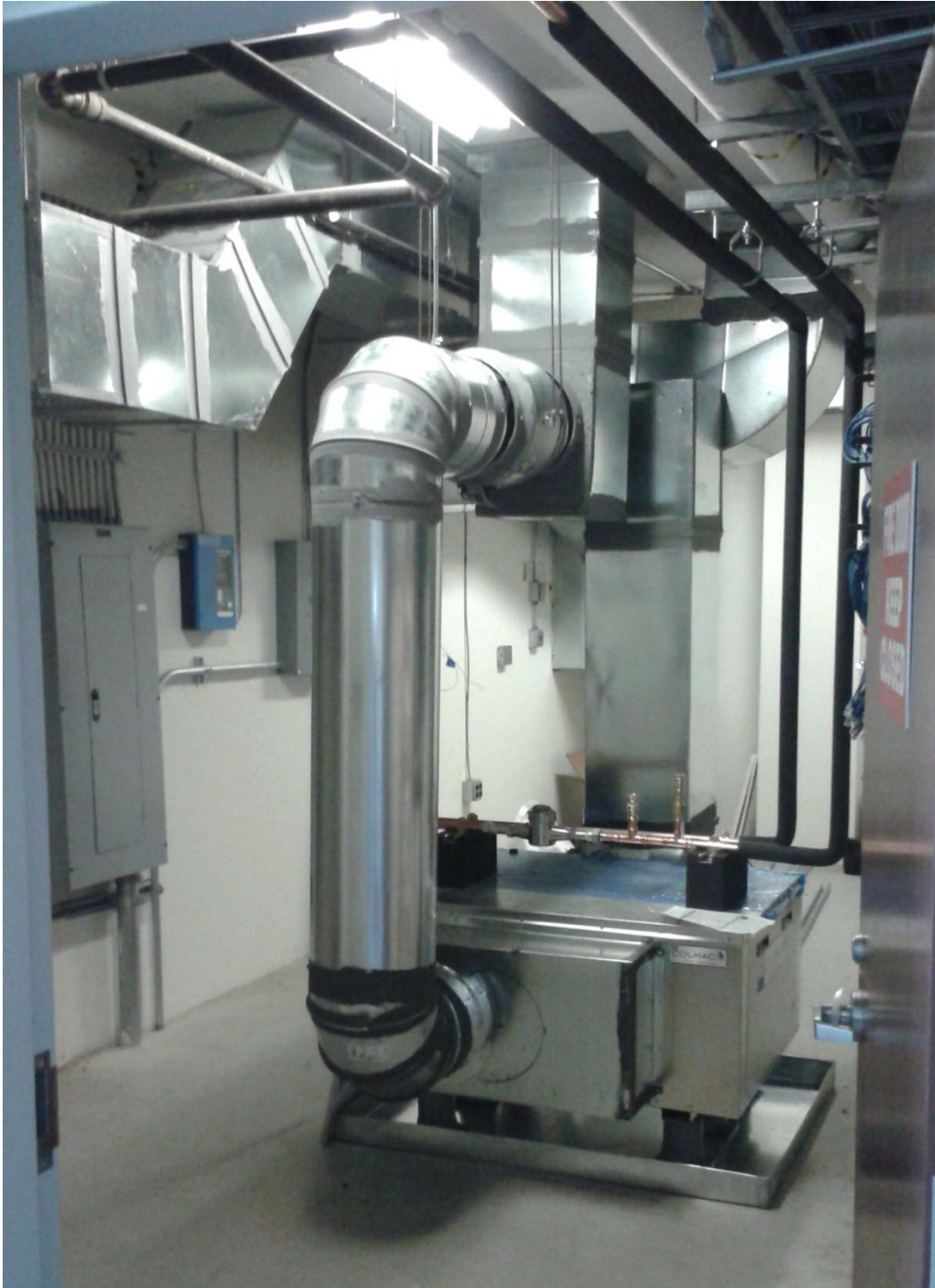
Figure 21. Heat Pump from Inlet Air Side
