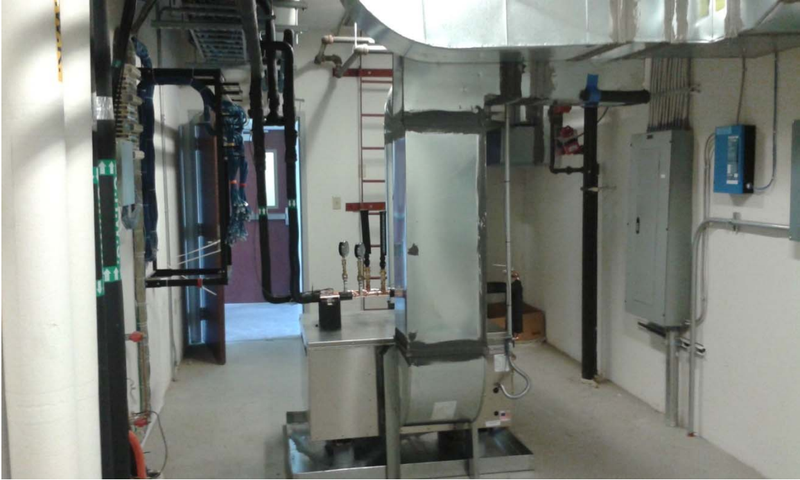
Figure 22. Heat Pump from Air Outlet Side
