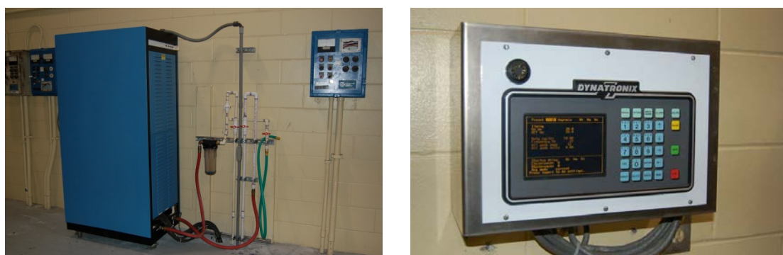
Figure 5-4. Pulse Rectifier with filtered water system (left) and MicroTouch Remote (right).
