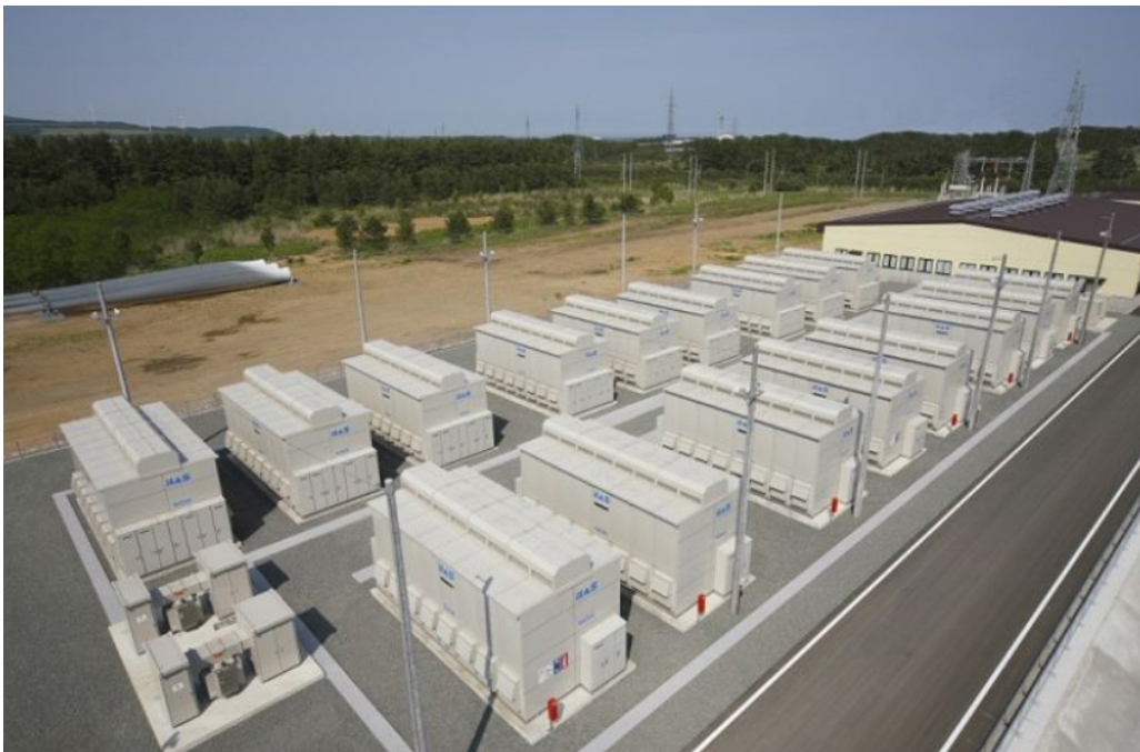
Figure 11. Sample Battery Storage Bank 115
