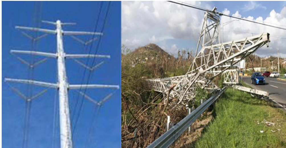
Figure 9. Collapsed Transmission Tower in Puerto Rico 101
