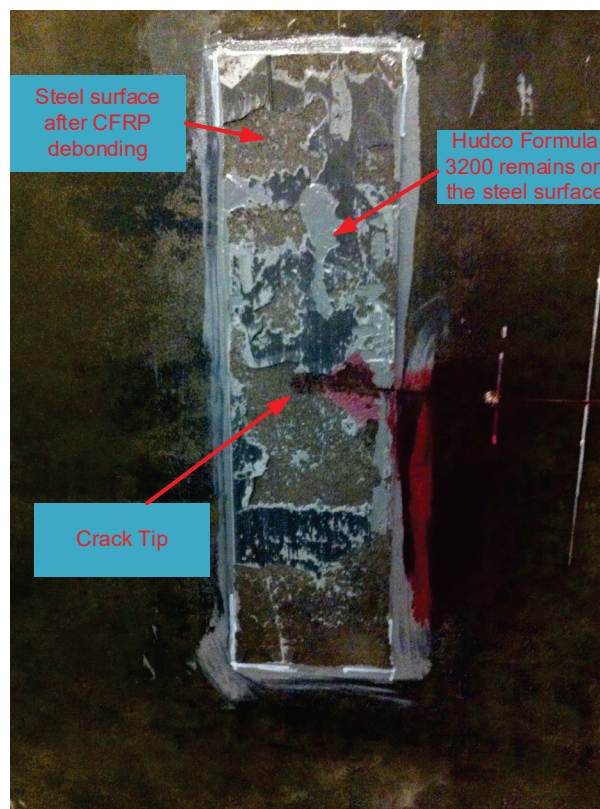
Figure 46. Steel surface after CFRP debonding (front left) at 378,756 cycles for Specimen 2.
