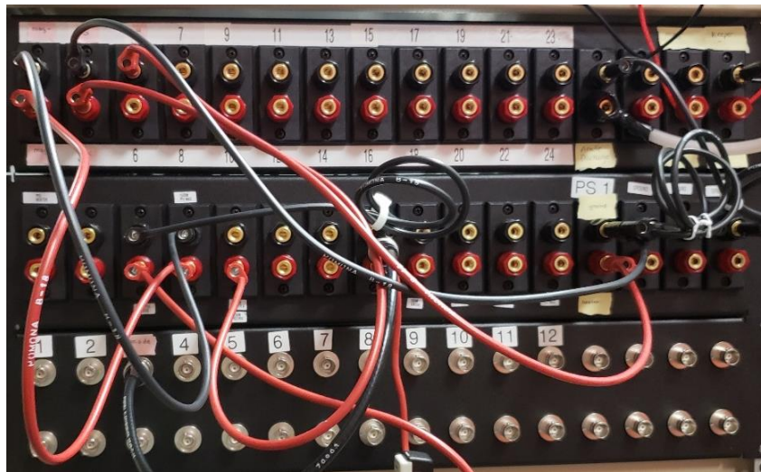
Figure 20. Banana Plug and BNC Electrical Connections Rack
