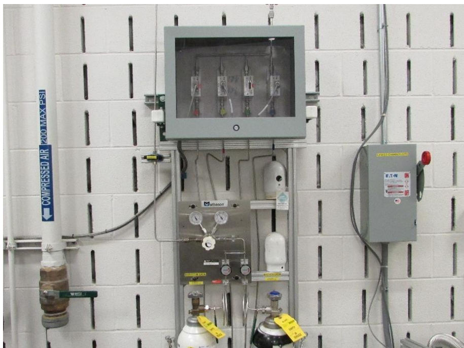
Figure 13. Propellant Line Plumbing
