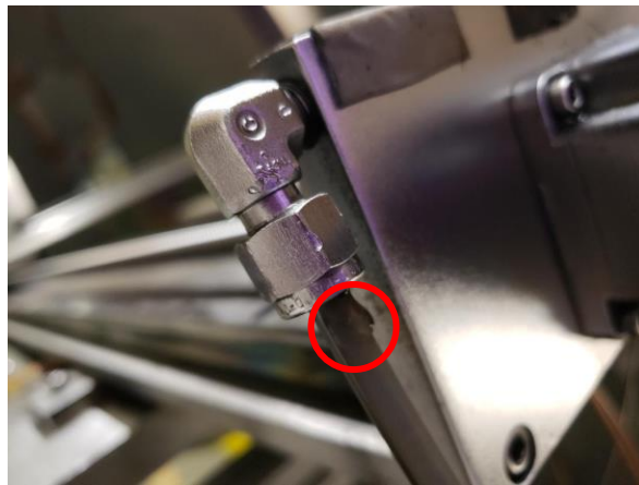
Figure 34. Water Leak from Traverse Cooling System Inside Chamber
