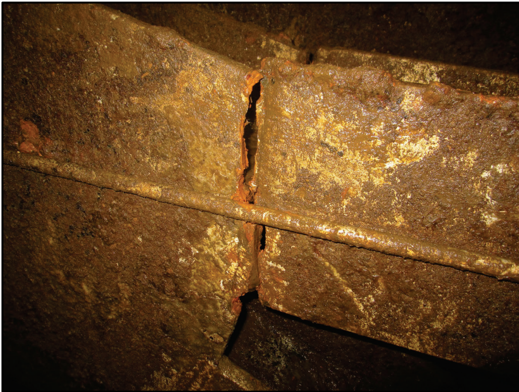
Figure 3. Crack found in gusseted plate on valve, September 2016.
