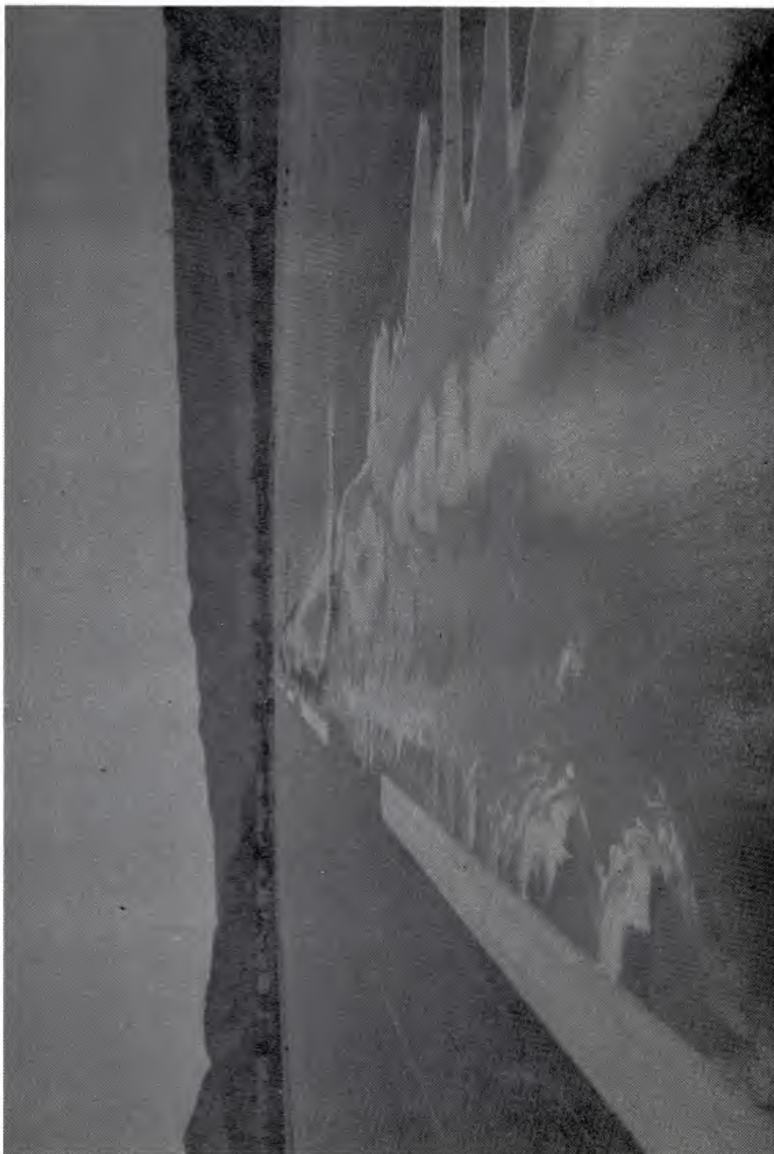
FIGURE 8. PONDED WATER REMAINING IN TEST SECTION 2 TWENTY MINUTES AFTER WATER APPLICATION
