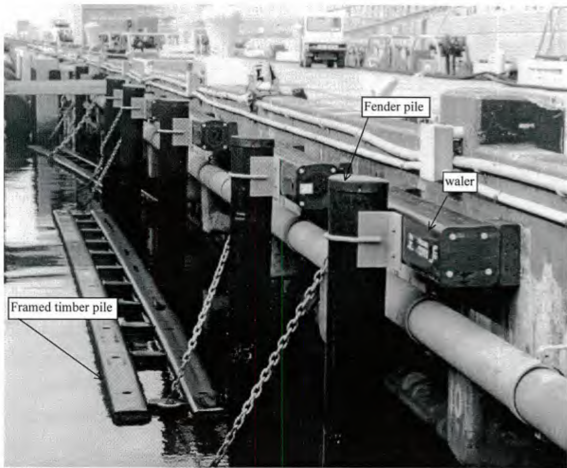
FIGURE 5. PLASTIC FENDER SYSTEM
