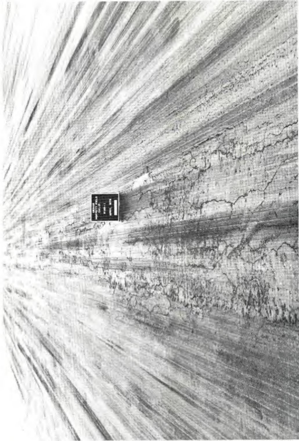
Figure 3. Pattern cracking, Discrete Area R14R-1.
