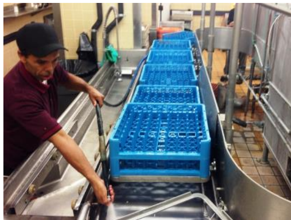
Figure 23. Pre-Rinse Station in Dish Room
