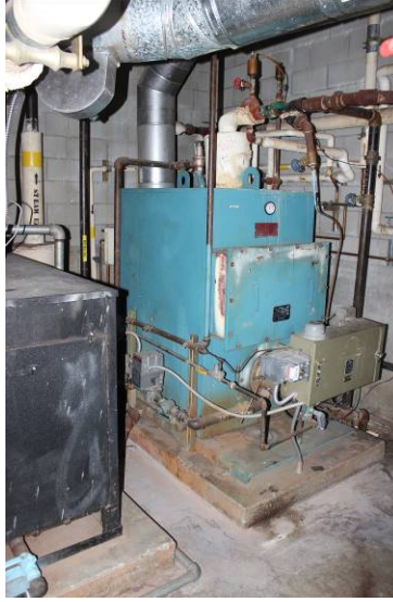
Figure 24. Boiler System for Decommissioning in DFAC
