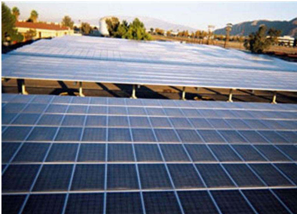
Figure 1: Photovoltaic array on two carports at March Air Reserve Base [13]
