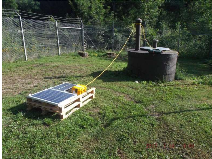
Figure 12: Grid connected test system, Spangdahlem Air Base, Germany
