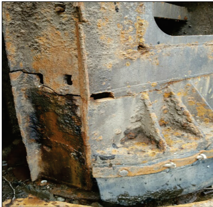
Figure 9. Cracking in the pintle area of a miter gate at the Captain Anthony Meldahl Locks and Dam.
