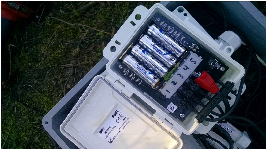
Figure 3.11: Data Logger Damage from Corrosion
