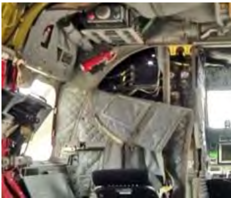
Cargo compartment fire extinguisher
