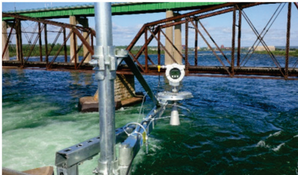
Figure 6. Upstream radar gauge placed on a Comp Works Gate 14.
