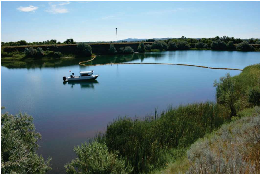
Figure 3. DC-1 after installation of the barrier curtain in July 2014 in Dredge Cut 2 at Fort Peck Lake, MT.
