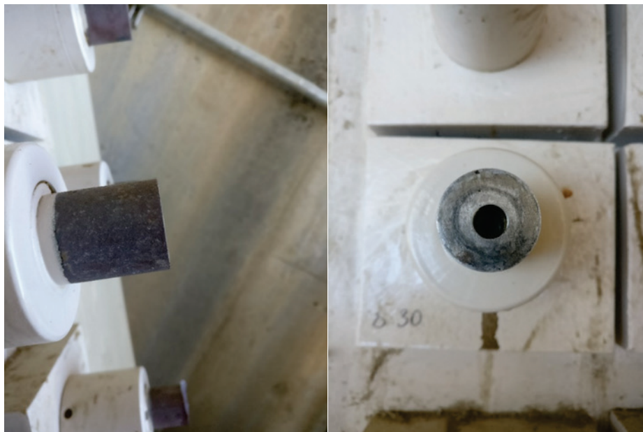
Figure 7. Oroville Dam rod condition.
