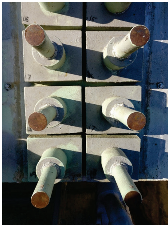
Figure 29. Pyramid Dam rod condition.
