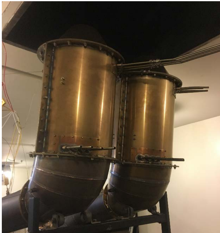
Figure 4. Heat Exchangers Installed on Engine Exhaust
