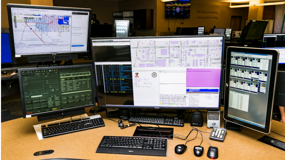
Figure 2. Multi-screen Dispatch Console
