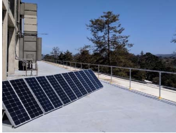
Figure 110. Setup of the PV panels.
