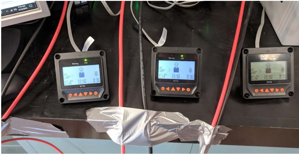
Figure 80. Remote meters monitoring in real time.
