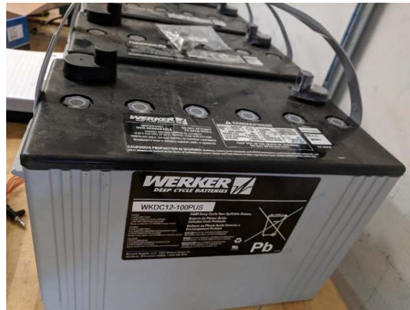
Figure 75. 12V-100Ah sealed deep cycle lead acid batteries.
