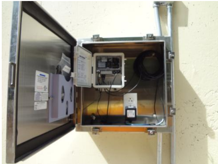
Figure C10. Data logger in a stainless steel weatherproof enclosure outside of ECM 12AC20.
