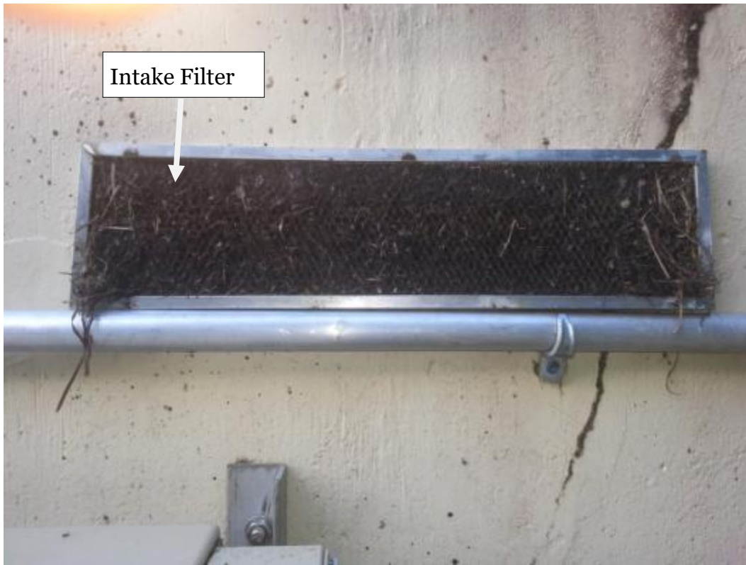
Figure 11. Clogged intake filter (removed for photograph).
