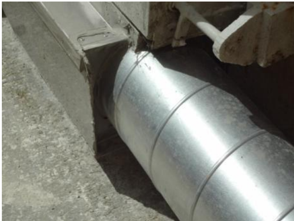
Figure C6. Stainless steel ducting connecting DH unit to ECM air input.
