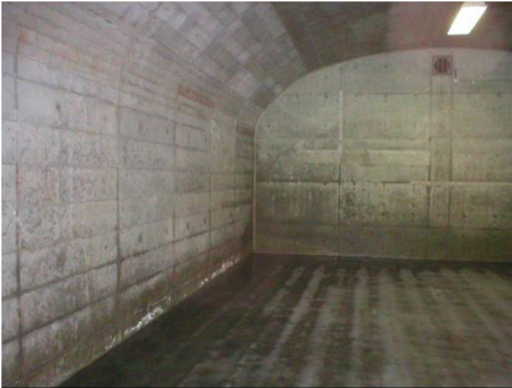
Figure 2. Water intrusion on floor, at left and background, in ECM 12AC20 at Guam.
