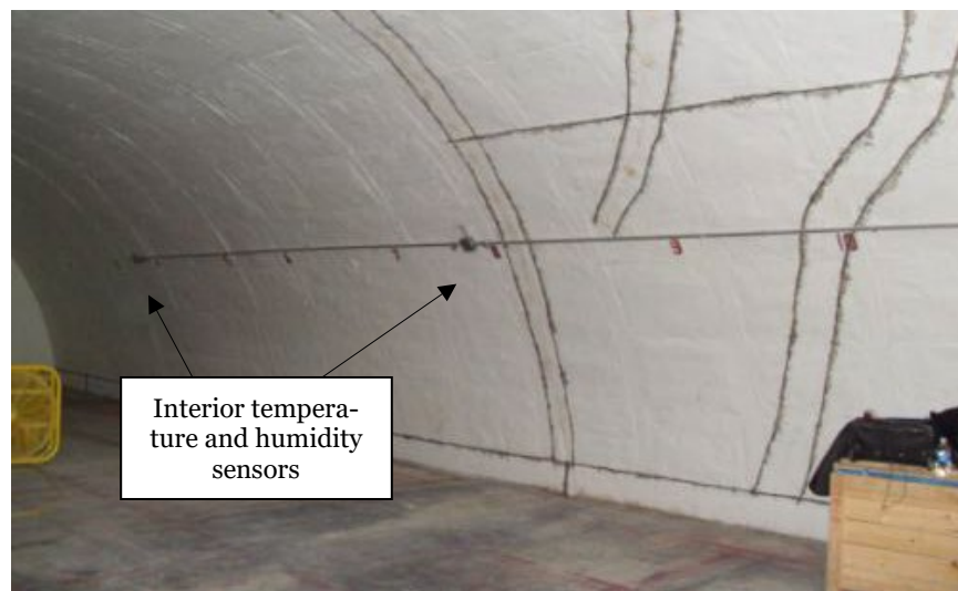
Figure C8. Wall-mounted sensors in ECM 12AC20.
