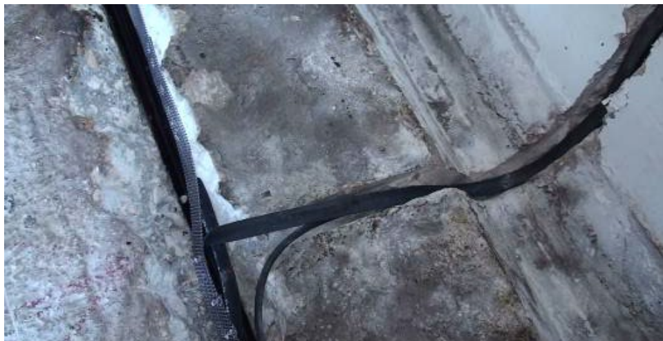
Figure A8. Floor anodes and lead wire.
