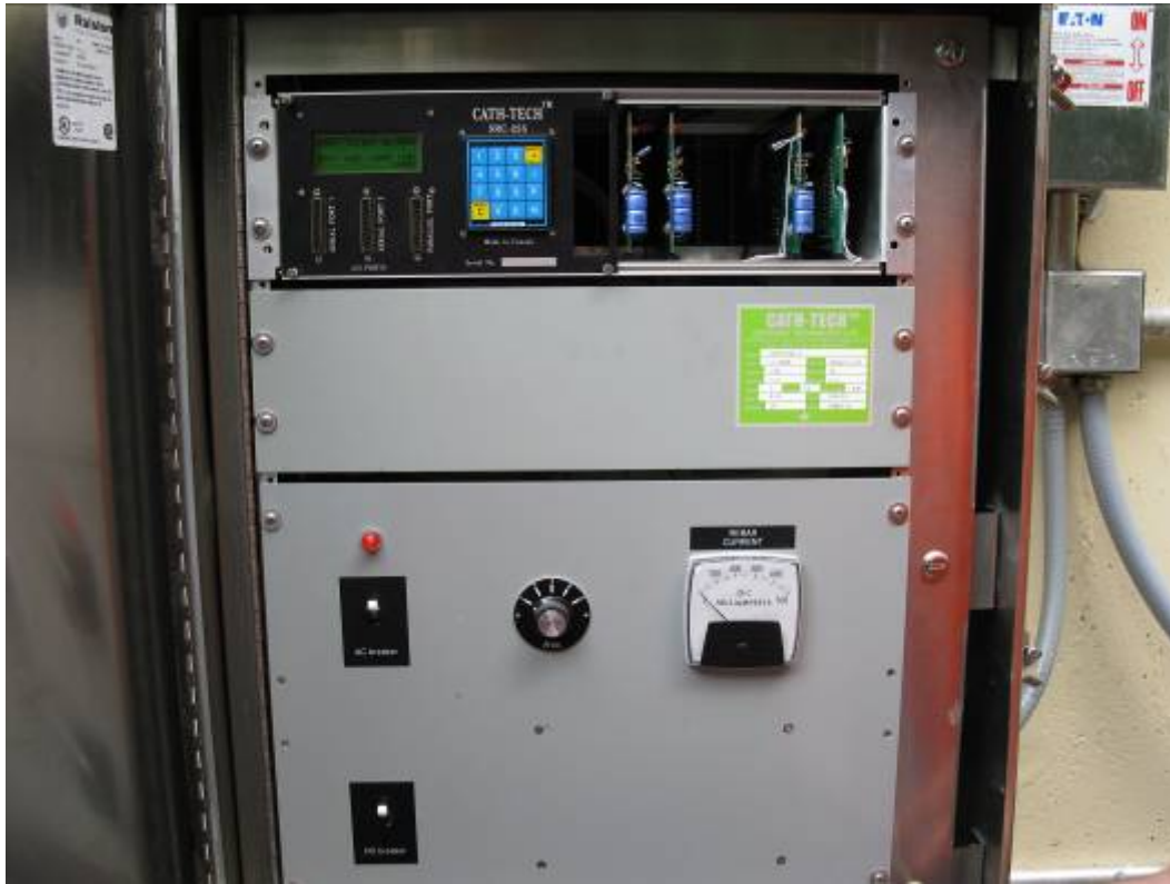
Figure A2. MCU main panel.
