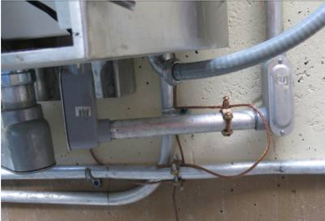
Figure A3. Galvanized conduit and junction boxes.
