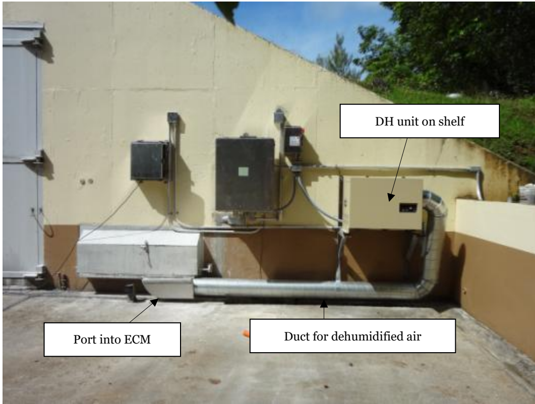
Figure C5. DH equipment installed at Guam ECM 12AC20.
