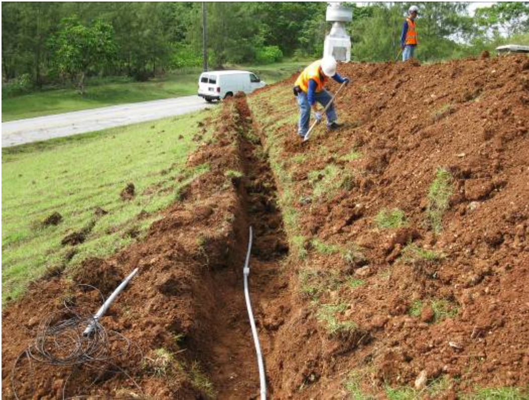
Figure A11. Cathode PVC conduit in trench.
