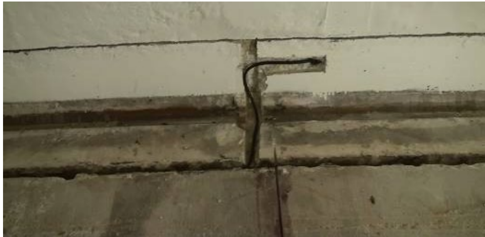
Figure A6. Moisture sensor.
