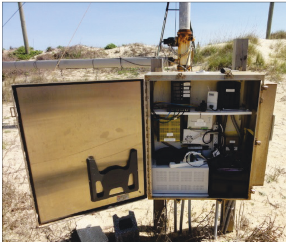
Figure 2-9. Lidar tower control cabinet.
