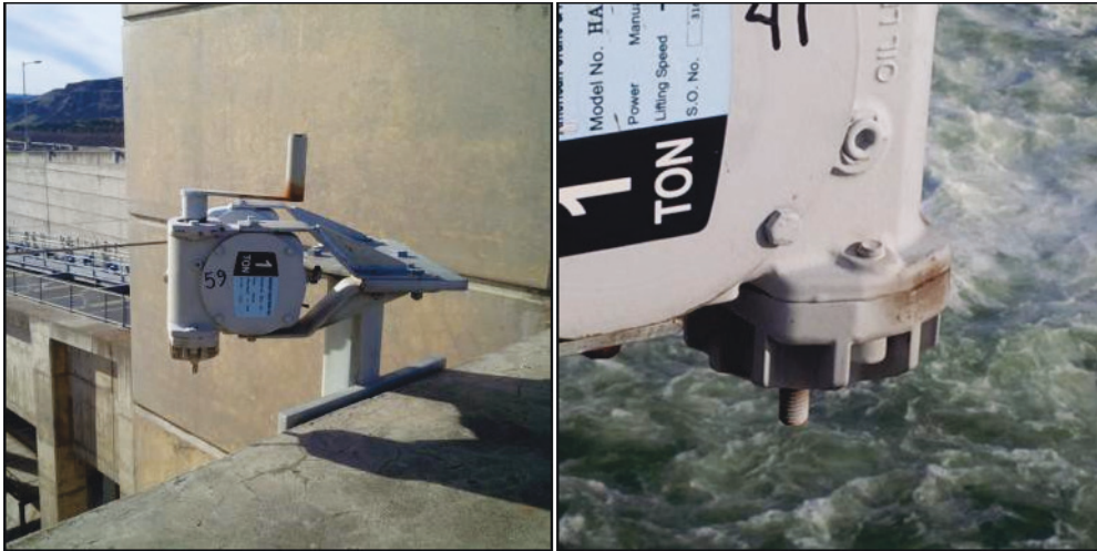
Figure 29. Cable ratchets at John Day Dam.
