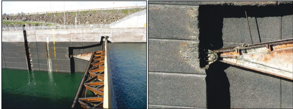
Figure 20. Upper Tainter gate at The Dalles Dam.
