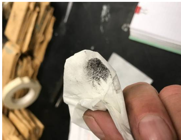
Fig. 5 Photo showing heavy smutting present on stainless steel panels
