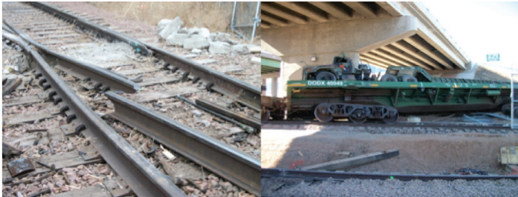
Figure 3.6 Damage from the 2011 Fort Carson Derailment
