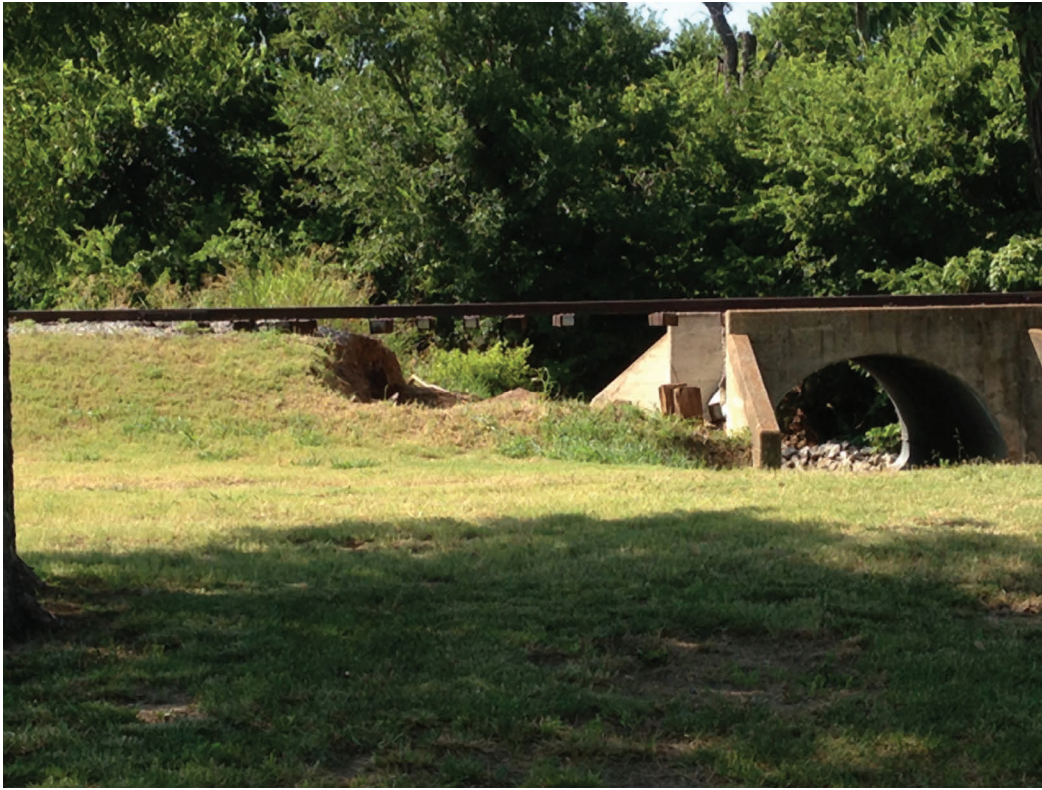
Figure 2.7 Photo of Fort Sill Track Damage from 2016 Flood
