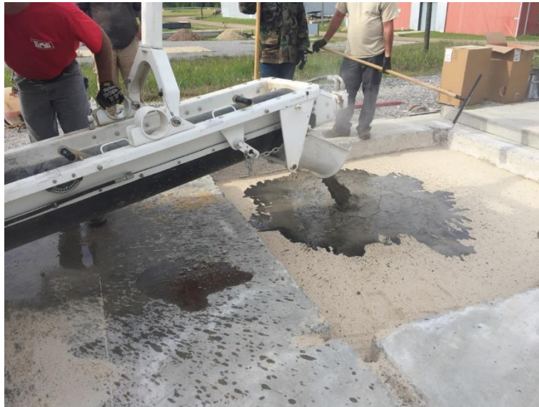
Figure 28. Excessive water initially delivered from volumetric mixer.
