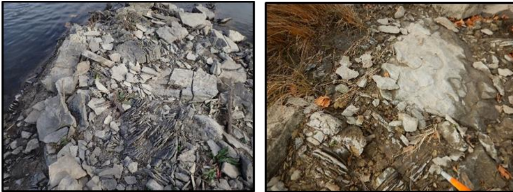
Figure 9. Weathering and degradation of bendway weir rock at RR1.
