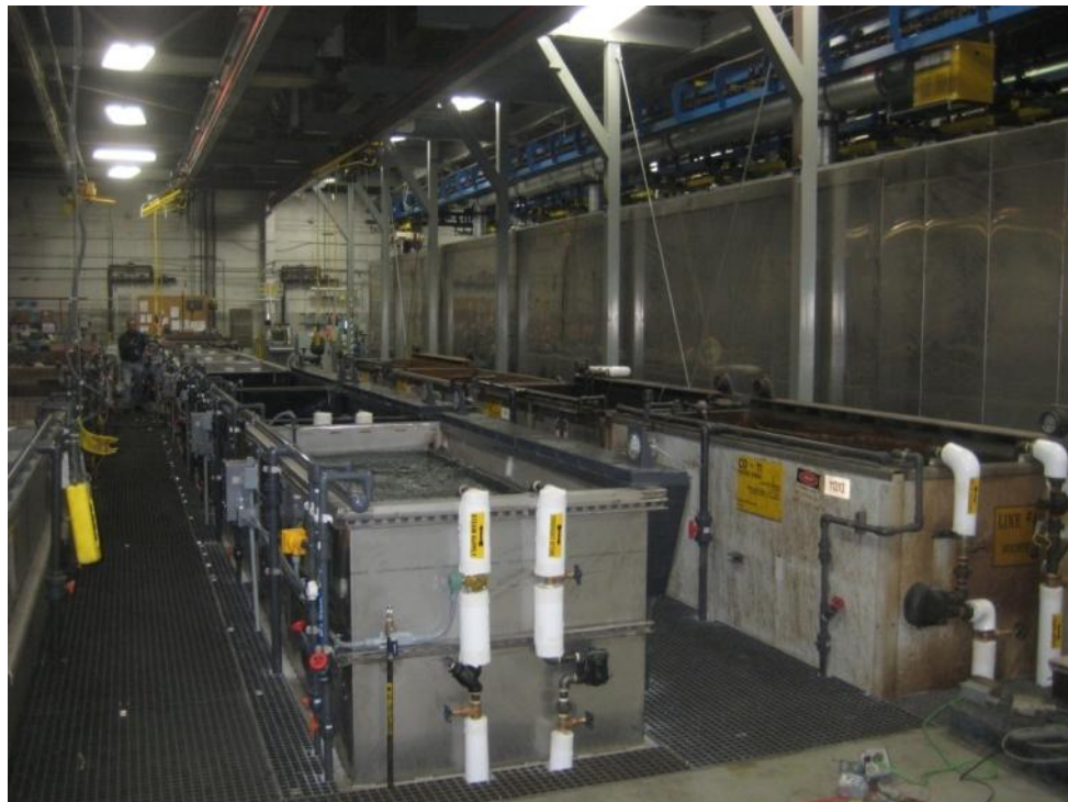
Figure 12: Installed Prototype LHE Zn-Ni Plating Line
