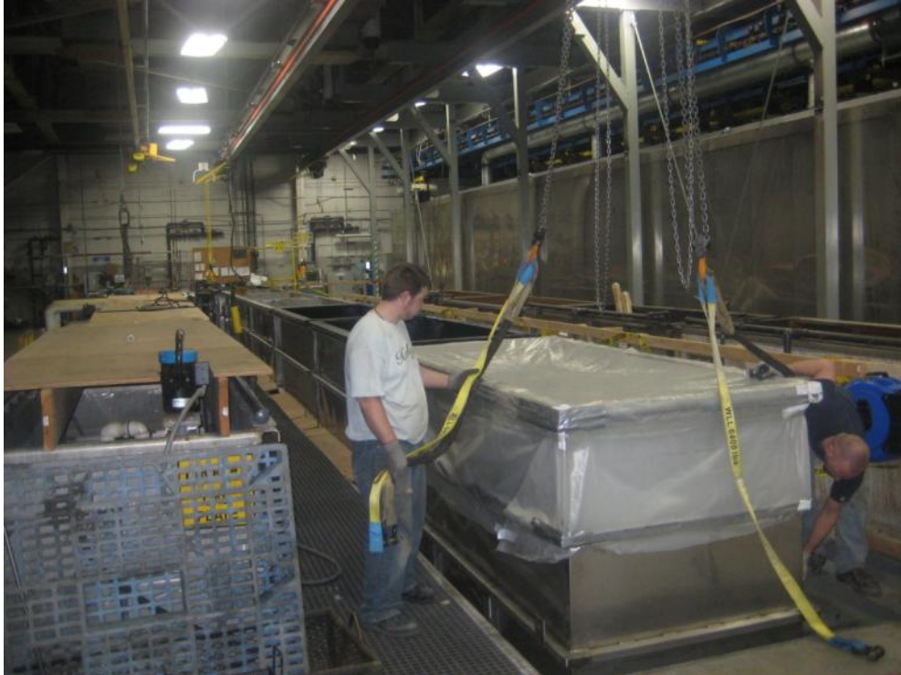
Figure 10: Prototype LHE Zn-Ni Plating Line Tank Installation
