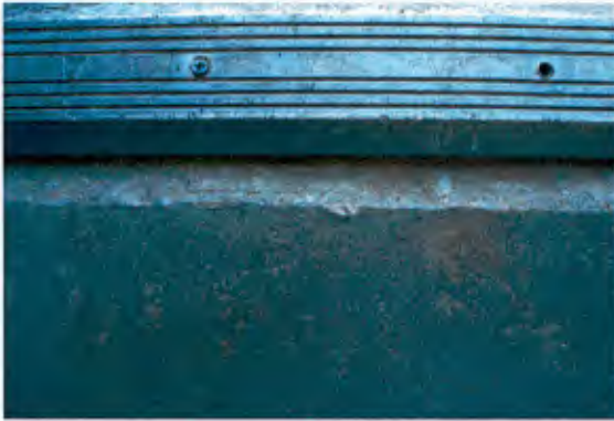
Keyed groove in area of heavy traffic.
