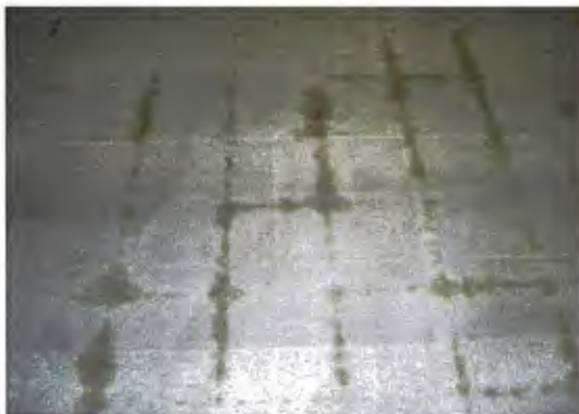
Shot blasted surface with oil contamination (Wet looking grid).
