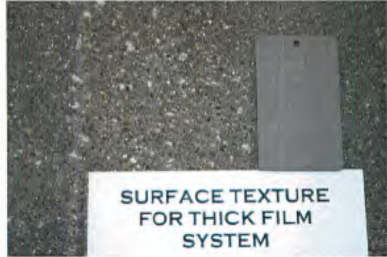
Two passes of shot blasting produced the above concrete profile (ICRI CSP 5).
