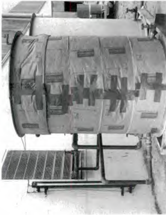
a. Blending and storage tanks (shown partially insulated).
