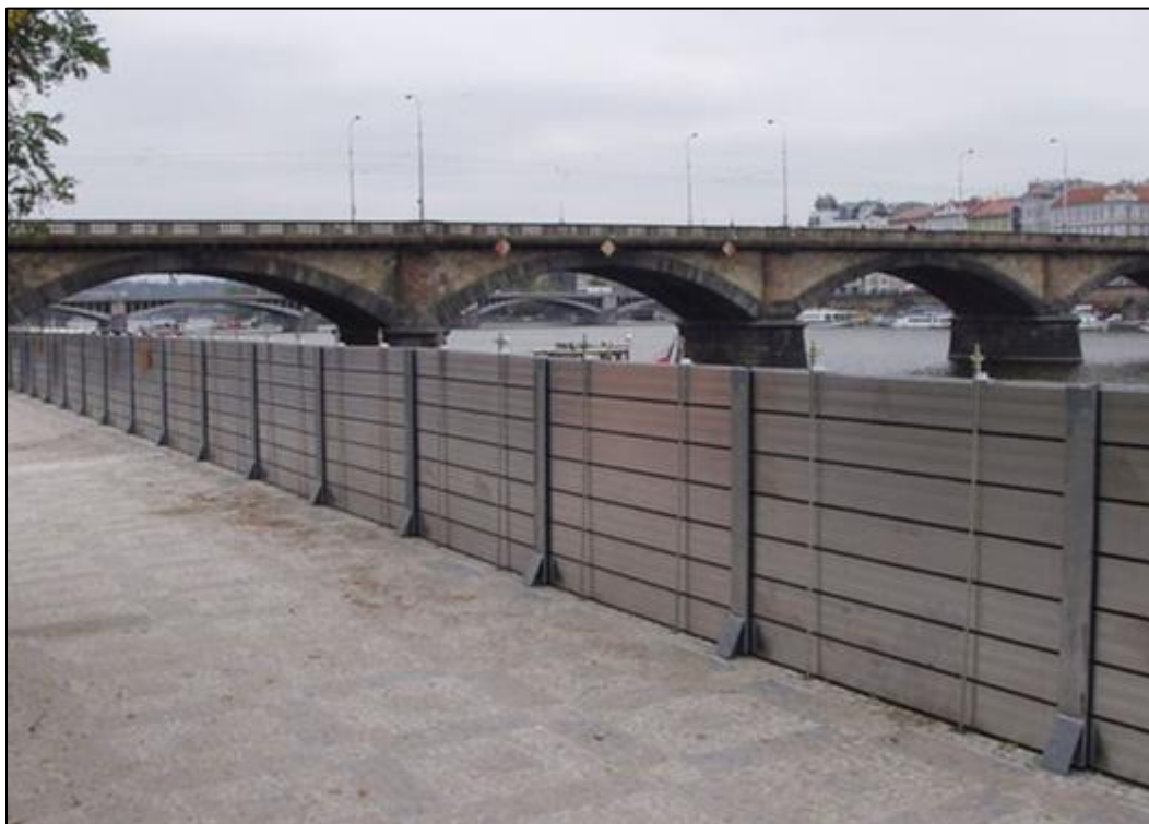
Figure 9. Demountable floodwall system.
