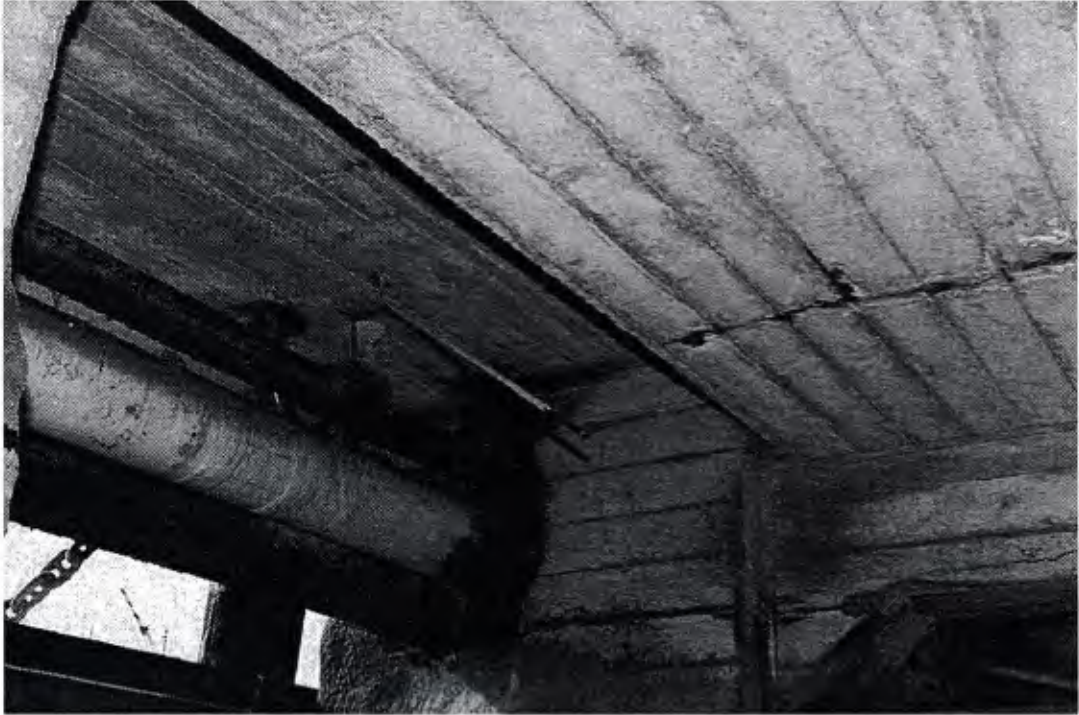
Figure 6. Deck underside at the thickness transition showing form marks (fins).
