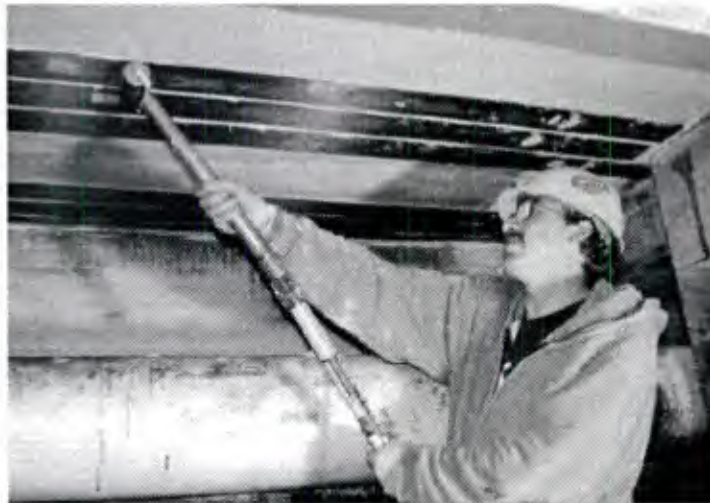
Figure 34. Installing pultruded carbon strips to the underside of the 8-inch deck section.
