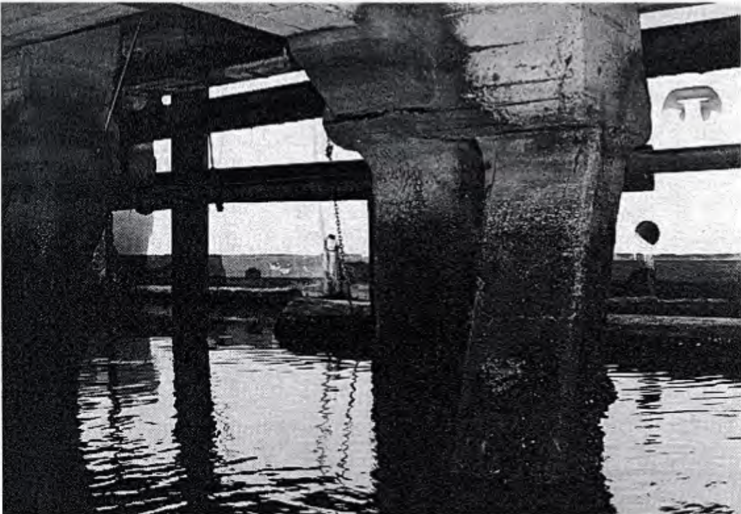
Figure 7. Marine fouling on vertical and batter piles under Pier 12.
