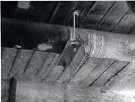
Figure 16. Fiberglass composite angle hanger at midspan between Bents 9 and 10.
