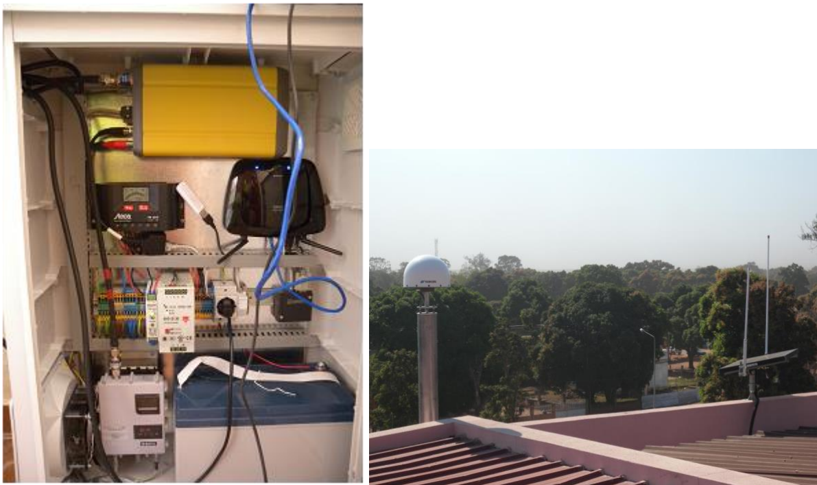
Figure 2 - Prototype developed for the integrated system. (left) cabinet hosting the equipment; (right) antenna monument and solar panels. Example of a system installed in Angola.
