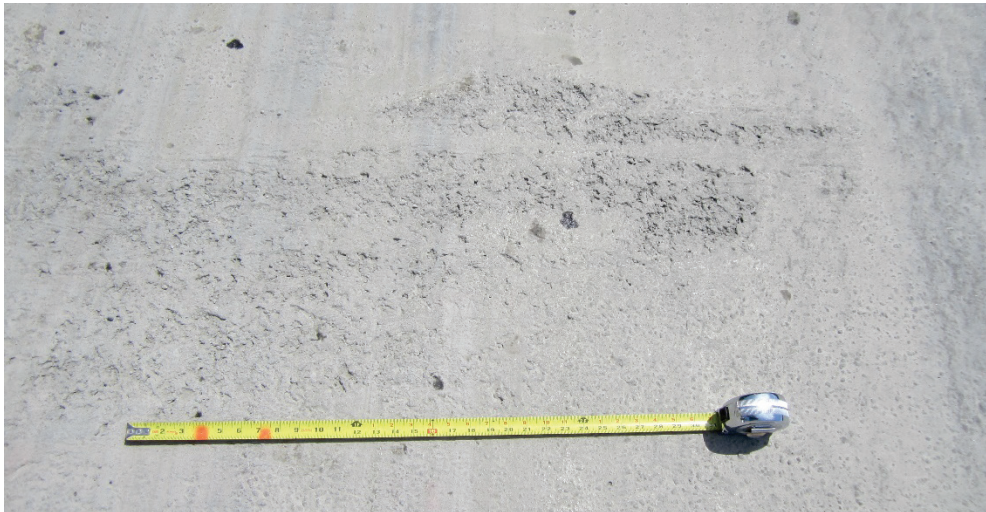
Figure 22. Repair 3, small rough area, 112 passes.
