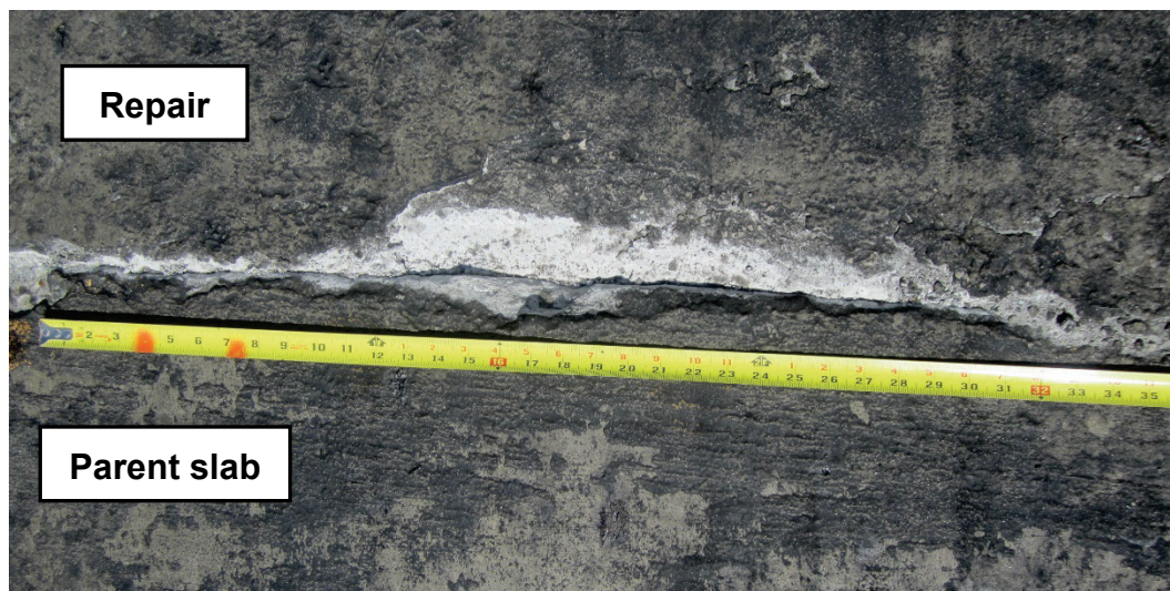
Figure 39. Repair 6, high-severity spalling, 3,500 passes
