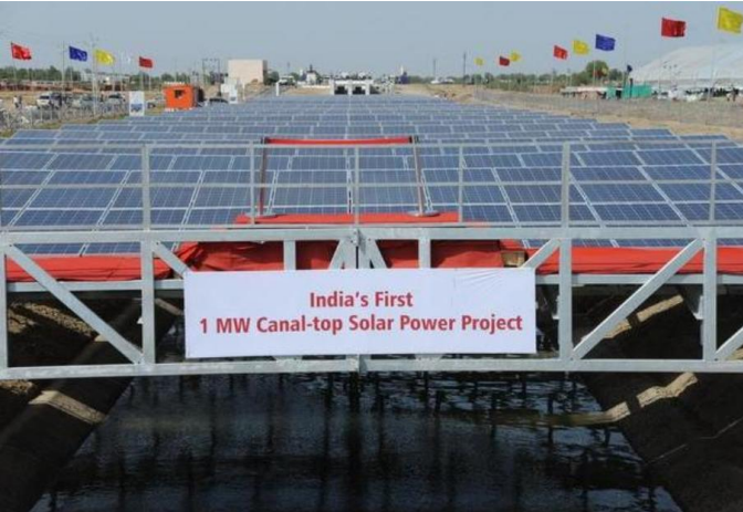
Canal Top Solar Power Plant
