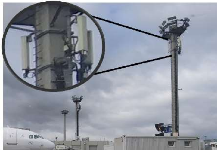
Figure 32 Cellular Antenna on a Floodlight above a Shelter at Frankfurt (Koser, 2020)
