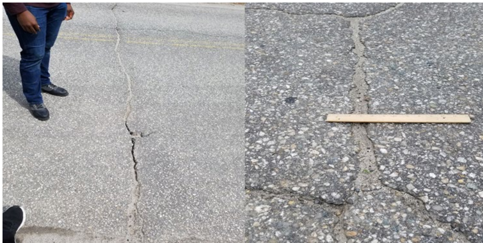
Figure 7. Corbin Road thermal cracking example in section 4.
