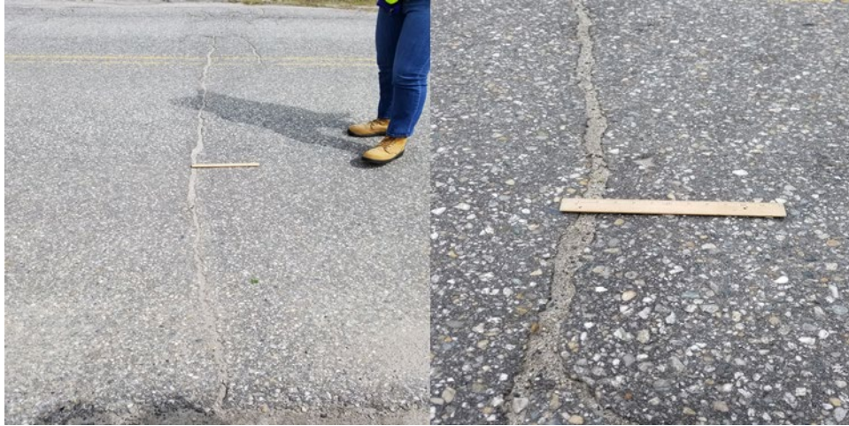
Figure 6. Corbin Road thermal cracking example in section 2.
