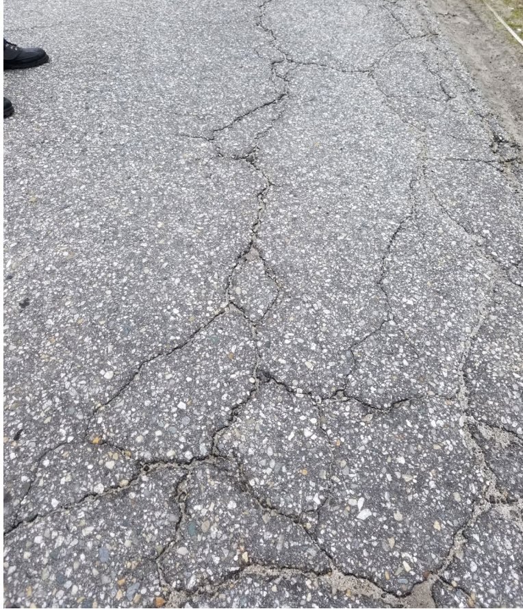
Figure 8. Corbin Road fatigue cracking example in section 4.
