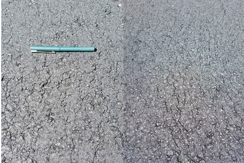
Figure 16. Check cracking observed in 2.5% polymer sections.
