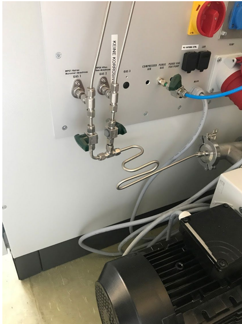
Fig. 2 Gas line pumping valves
