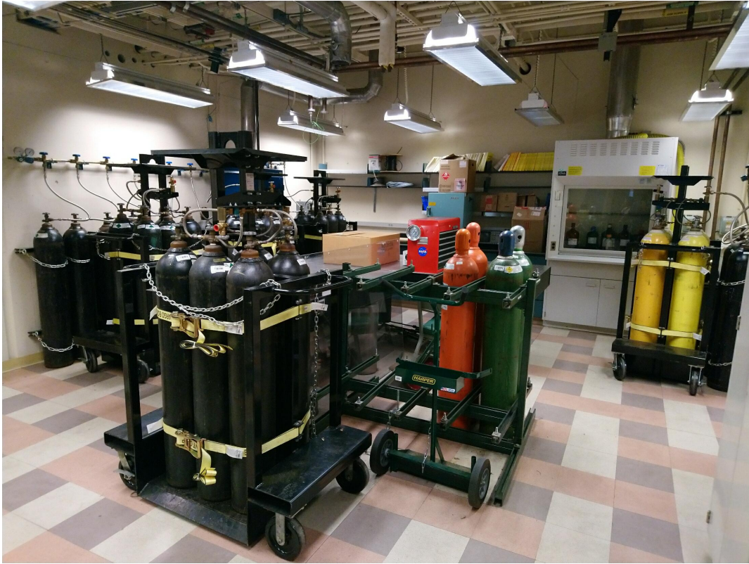
Figure 1: Photograph of previous gas-handling system
