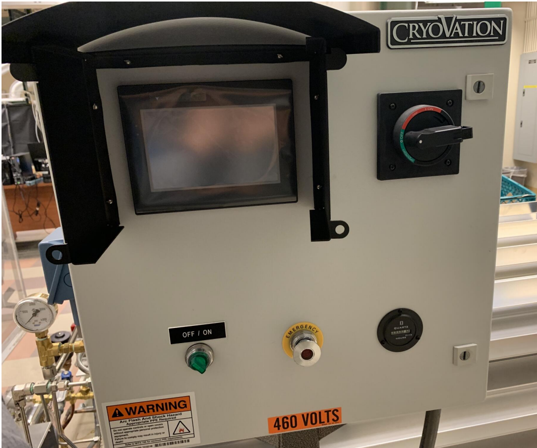
Figure 5: Photograph of the control panel.
