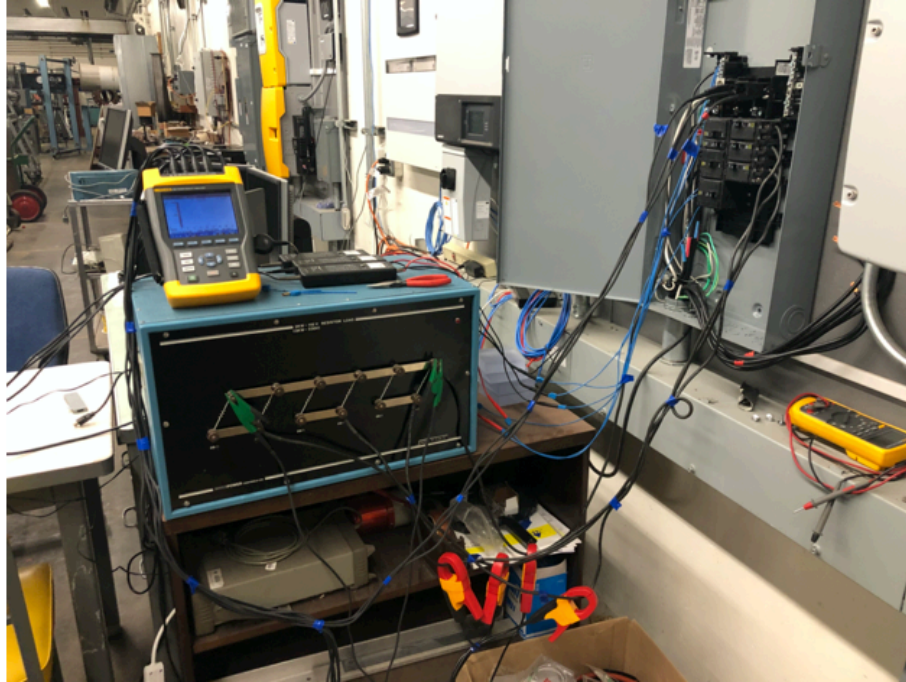
Figure 9. Microgrid Laboratory Breaker Panel Data Collection Setup
