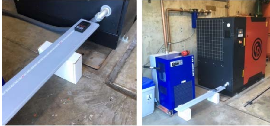
Figure 9. Testing Apparatus for 460V System
