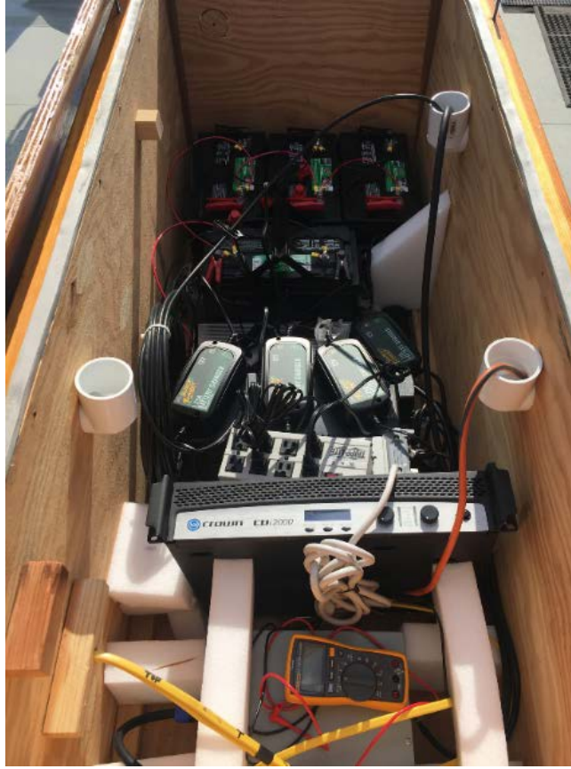
Electronic equipment inside the coffin which powered and delivered the signal to the source.
