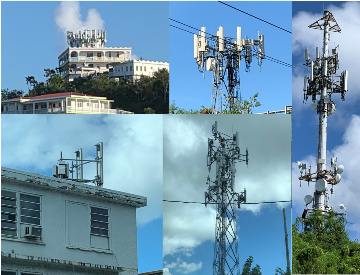
Figure 3.2. Examples of Cell Towers in the USVI.
