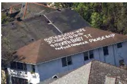
One of several messages left on the roof of a home shortly after rescue efforts began in New Orleans, La., in the wake of Hurricane Katrina, on Sept. 7, 2005. (U.S. Air Force photo by Tech. Sgt. Mike Buytas, 1st Combat Camera Squadron) 050907-F-9085B-023
