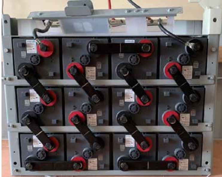
Figure 37. Battery Bank of Experiment
