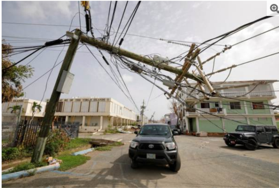
Figure 1.8. Hurricane Maria Damage on STX. Source: Reuters (2017).
