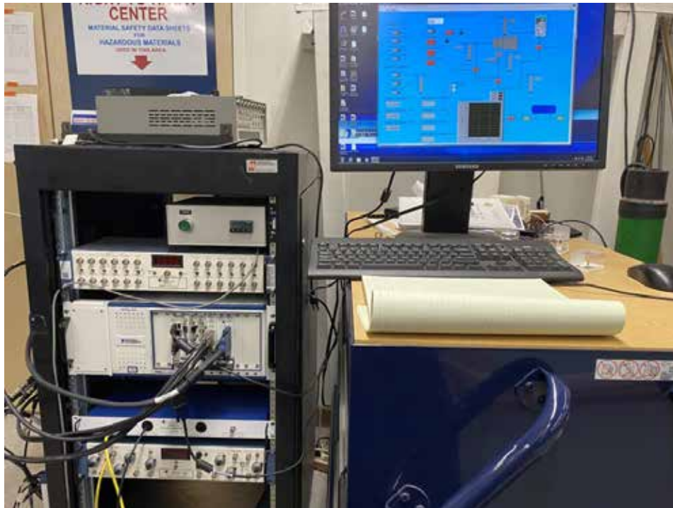
Figure 16. Valve and firing control system for the light gas gun.
