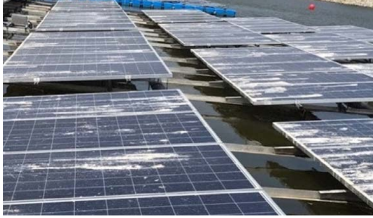
Figure 12. Soiling due to Bird Droppings. Source: [12].
